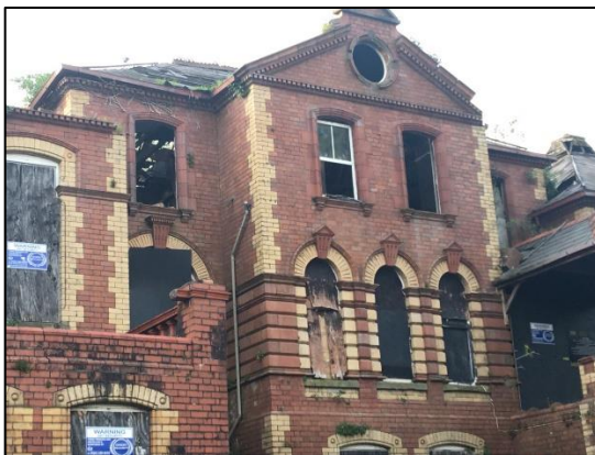
Photo 9 Missing tiles on southern elevation
