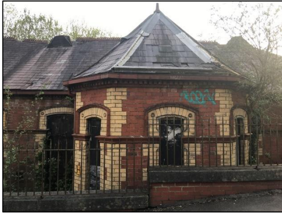
Photo 11 Missing tiles on eastern elevation
