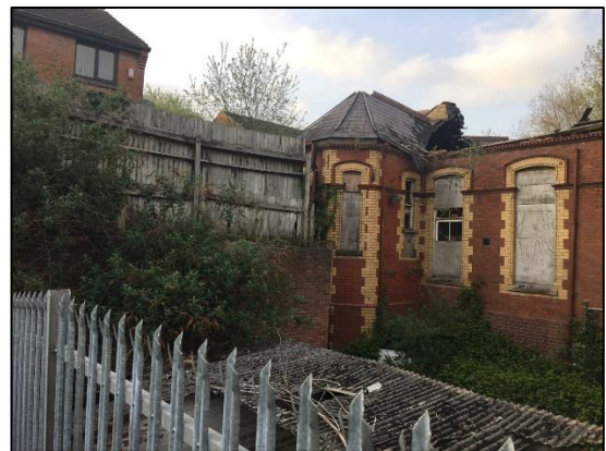
Photo 10 Missing tiles on western elevation
