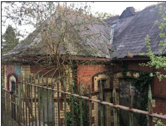
Photo 13 Missing tiles on eastern elevation
