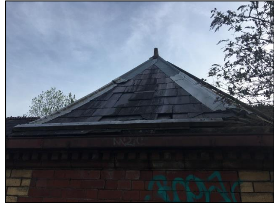
Photo 12 Missing tiles on eastern elevation
